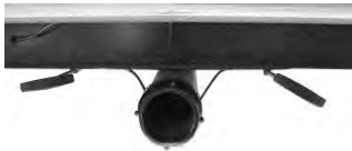
Black/Grey Tank Drain and Valves
