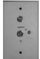
Antenna Power Supply
